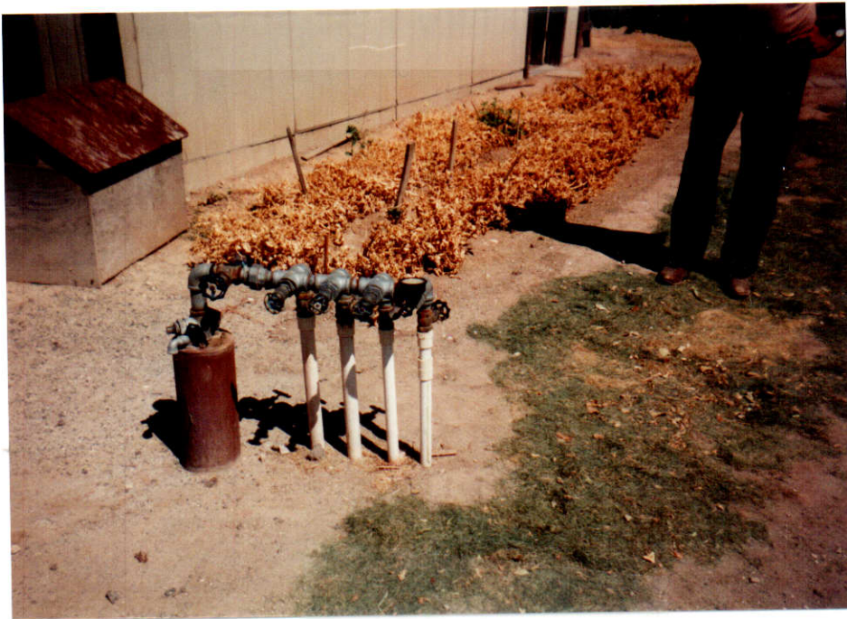
view of well & valves to the 4 circuits.
