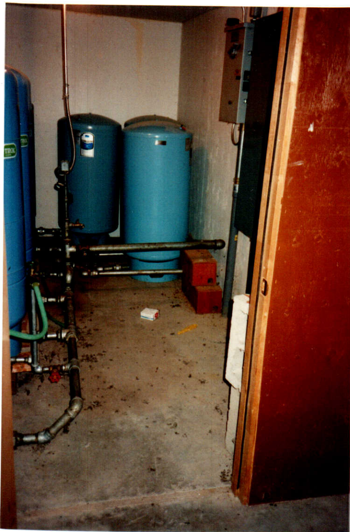
PHOTO #2 PRESSURE TANK AND PUMP CONTROLS INSIDE NORTHEAST CORNER OF IMPRINT BARN. MAIN LINE IS 2-INCH PIPE.
