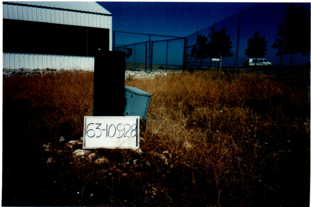
PHOTO #1 8-INCH WELL AND 15HP SUBMERGIBLE PUMP. IMPRINT BARN IN BACKGROUND.
