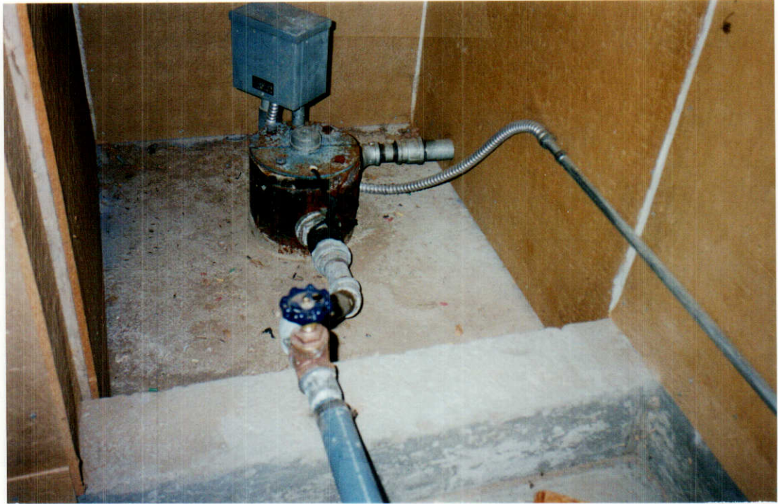
PHOTO ONE- well and irrigation service line exiting through well house wall.
