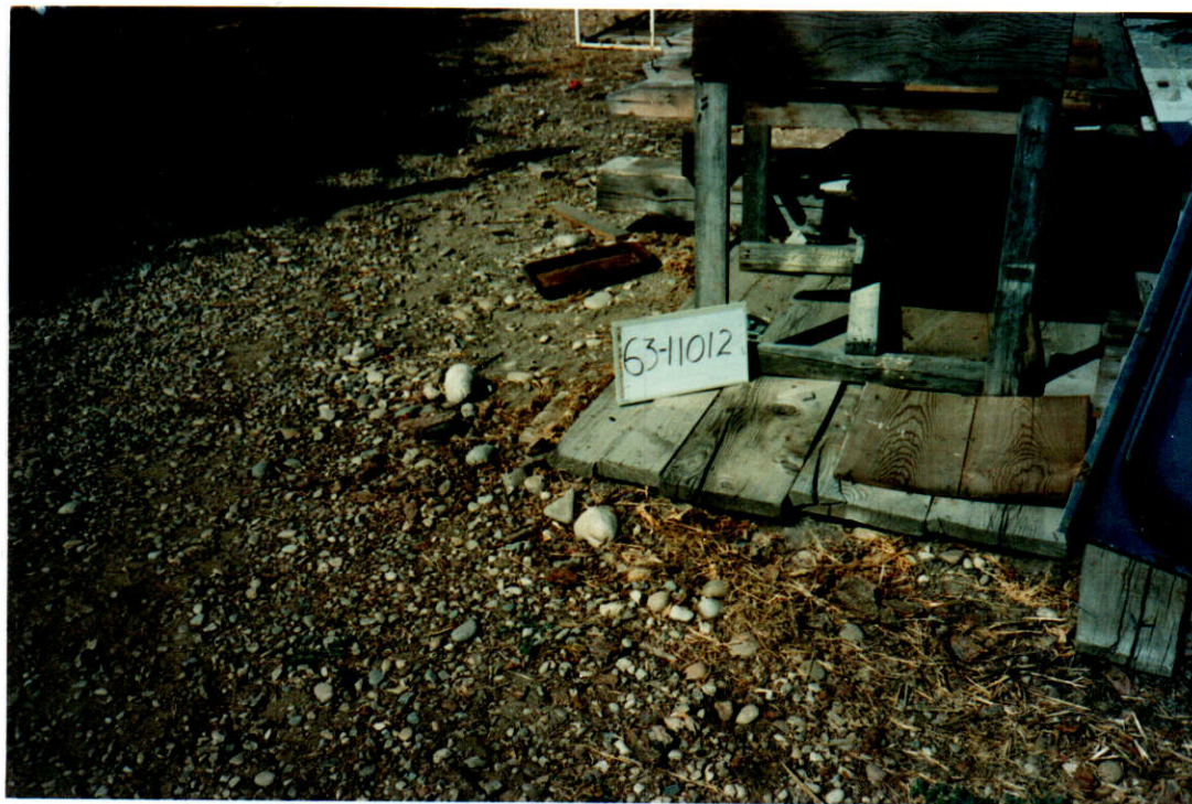
PERMIT 63-11012 PHOTO #1 15-INCH WELL EQUIPED WITH \frac{1}{2} HP CENTRIFUGAL PUMP.
