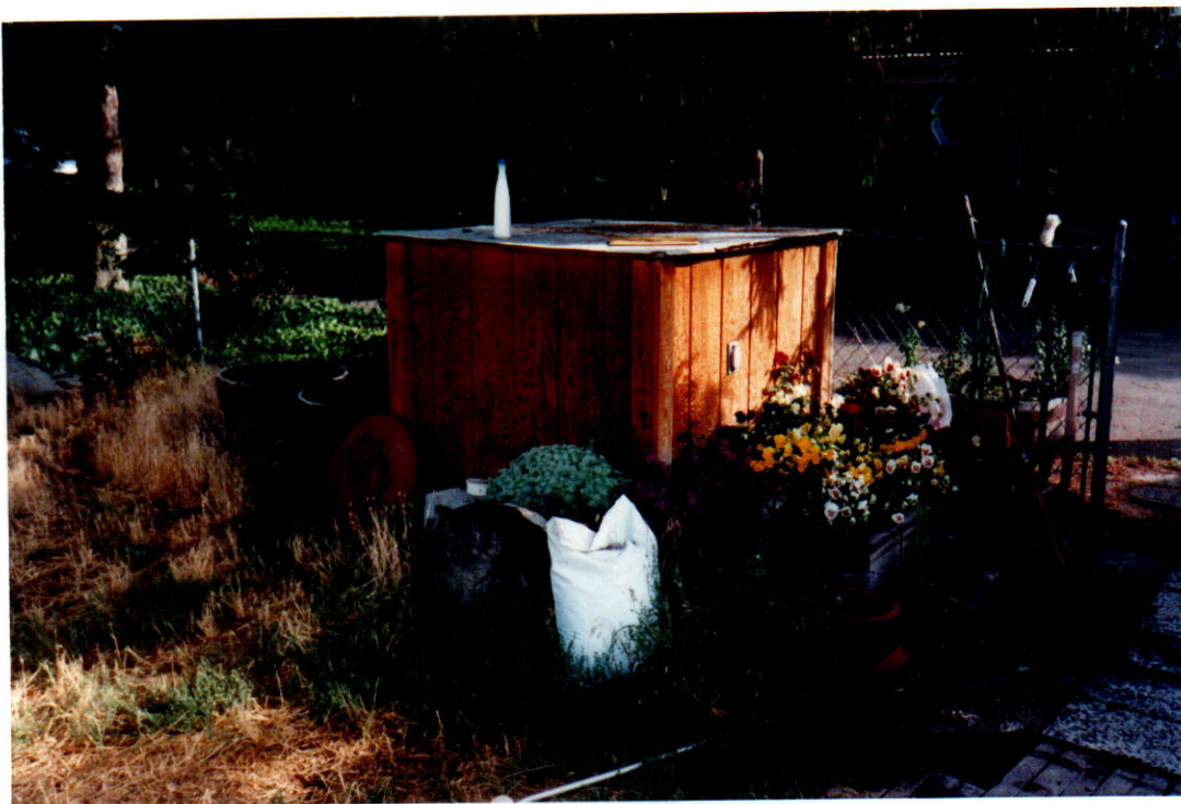
Pressure Tank Housing.
