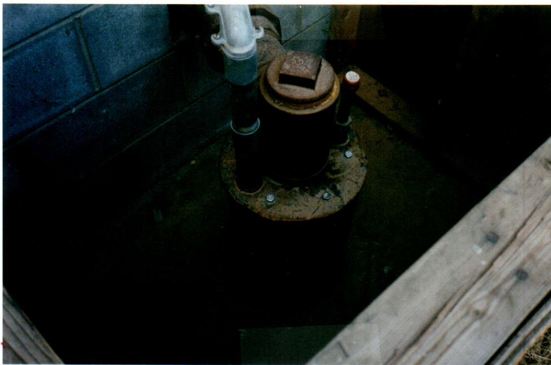
PHOTO TWO- Well with 10" casing inside small structure.
