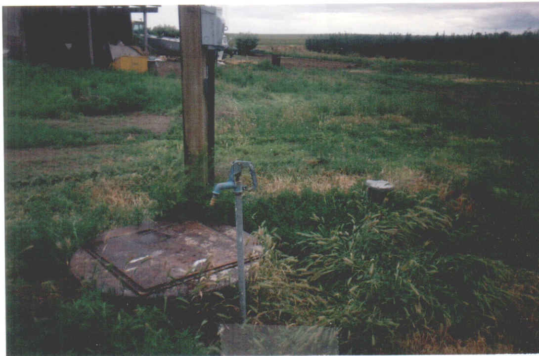
PHOTO ONE- Well And irrigation Valve control box Located west of home.
