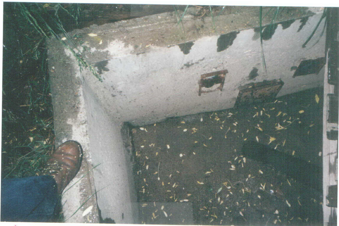
Irrigation Box located east of home across driveway. Three slide gates and a 4" PVC pipe are used to distribute water to lawn area and pasture.
