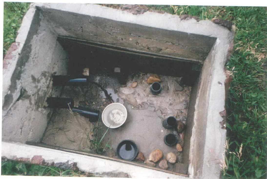
PHOTO THREE- Distribution box to distribute water through pipe to flood irrigate north and east portion of lawn.
