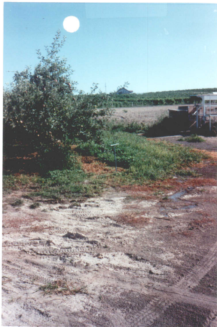
VALVE CONTROL FOR 2" PIPE SESESE, SEC 27 (WINERY in FOREGROUND)
