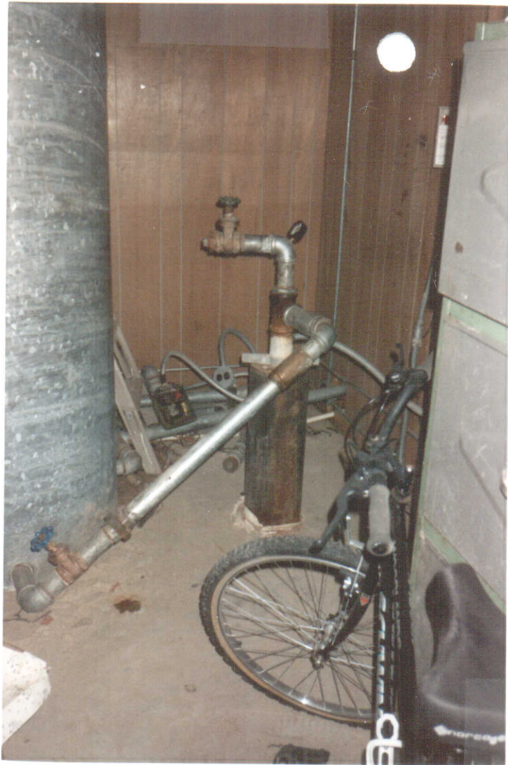
WELL #1, NESW, SEC 35 15 HP BERKELEY SUBMERSIBLE
