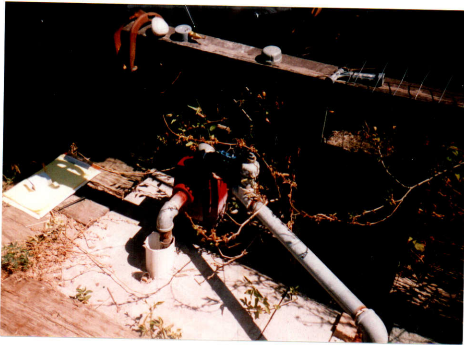
view of well, on north-east side of the house. pipes to the domestic use as well as the irrigation usage
