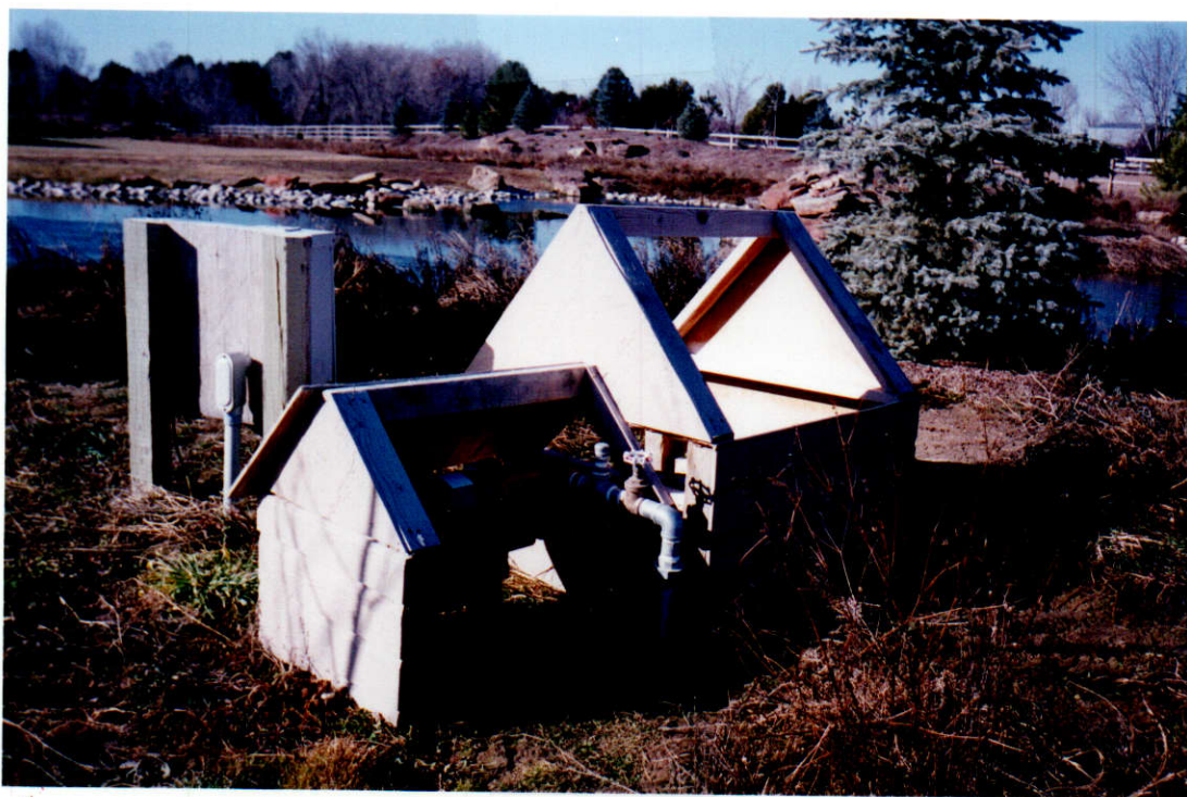
Irrigation pump and sump next to pond.
