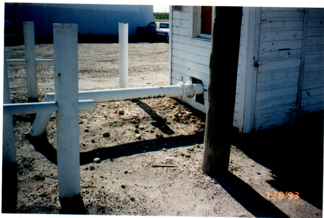
6" discharge into 8" main- line across rd - gravity/ Flood irrigation system.
