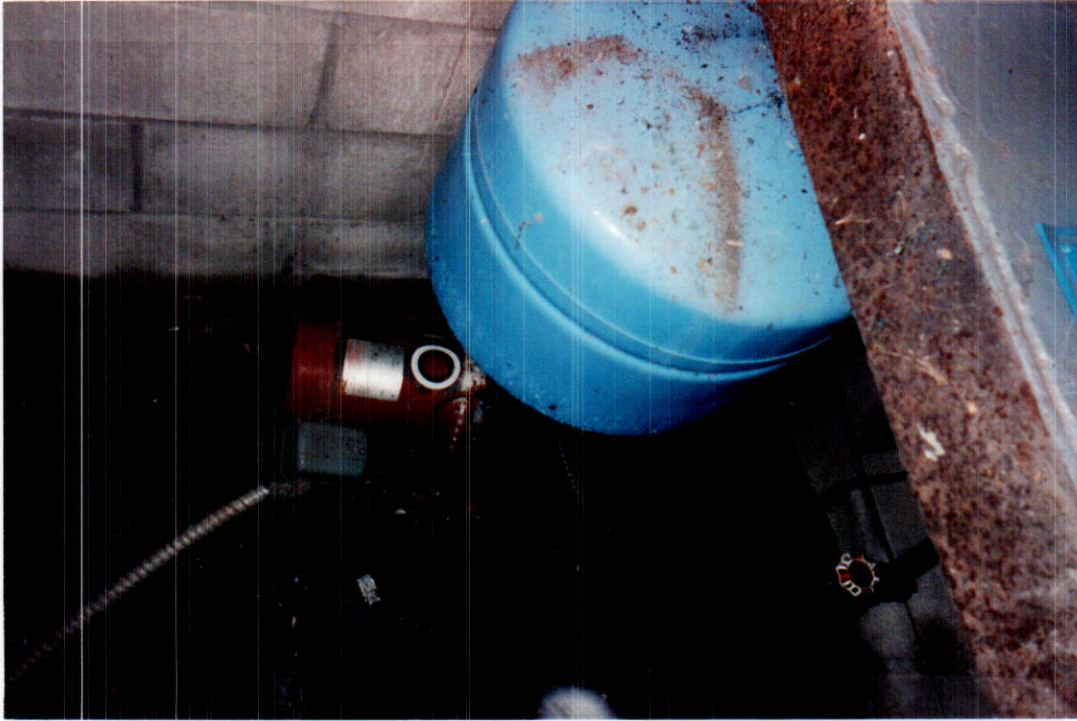
View of well Pump & Pressure tank. Located in the main building SHOP.
