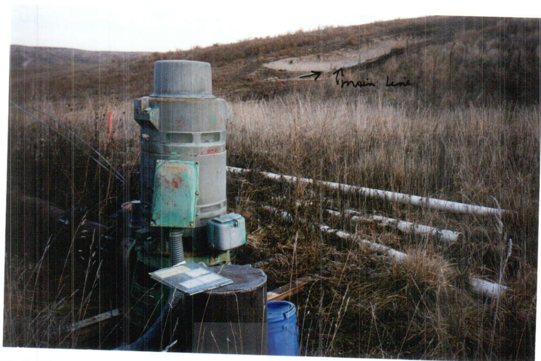
PHOTO THREE- View northeast of well No. 2, located in nwsu Sec. 1. 10" main line from pump, and 8" main line up hill.
