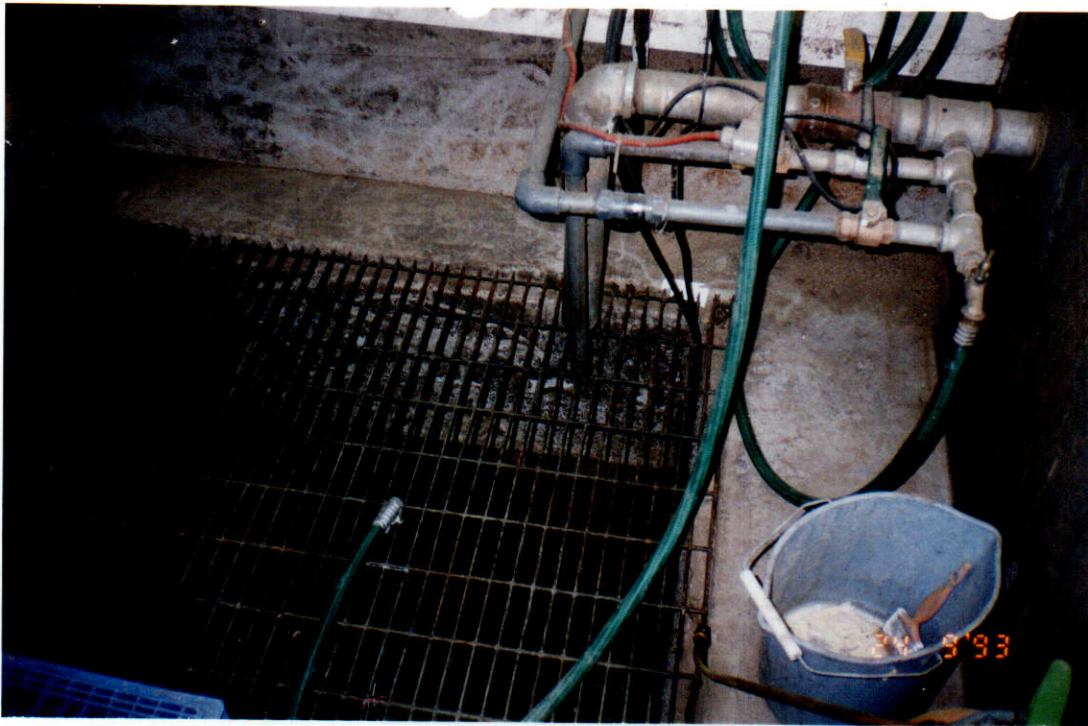
500 Gal cement holding tank for beet washing
