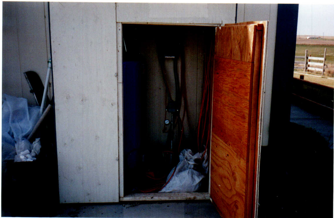
Pump house located on north side of home.
