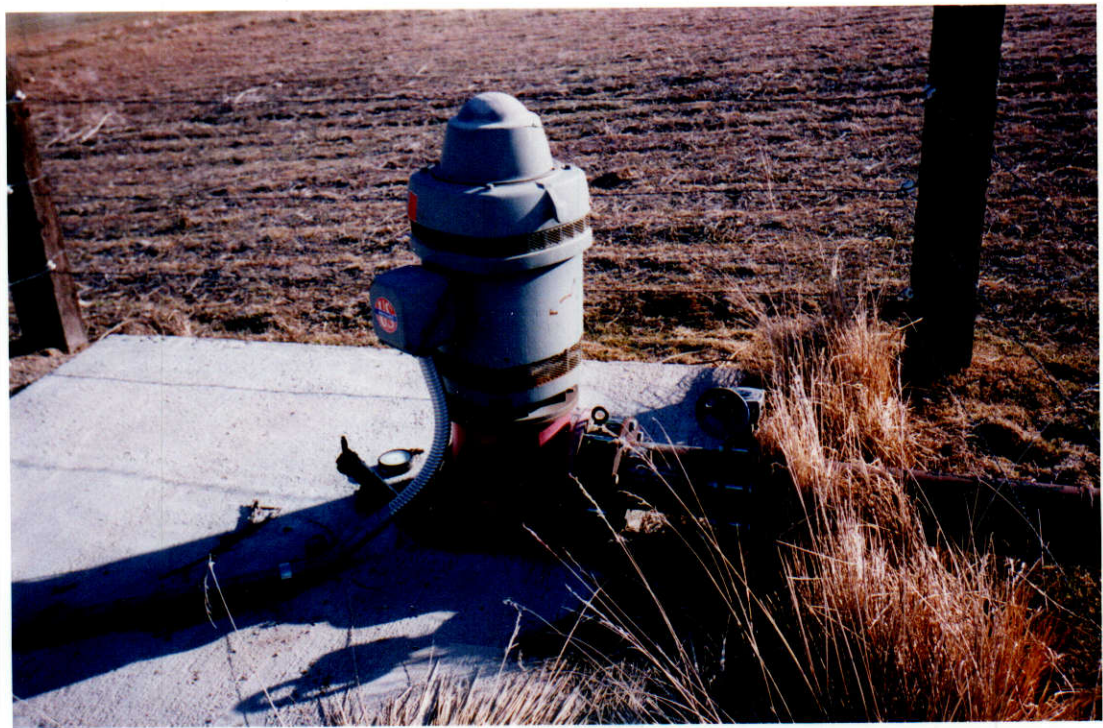
PHOTO ONE- well and 8" discharge line which leads to concrete irrigation ditch.
