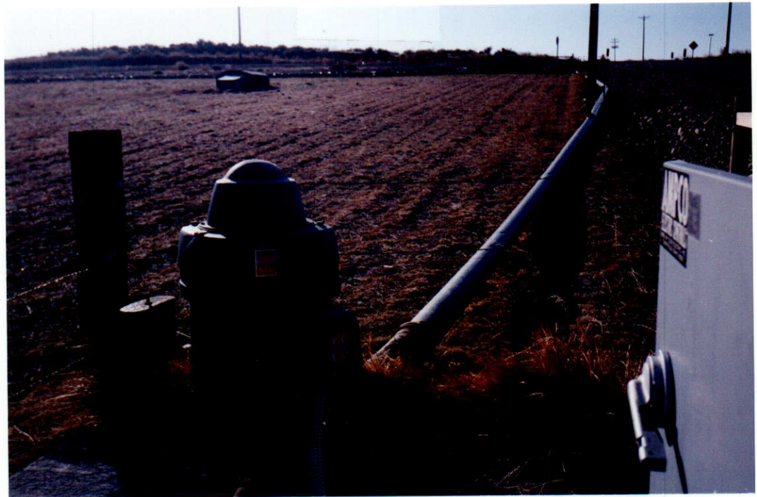
View southerly of well and 8" discharge line to upper concrete ditch.
