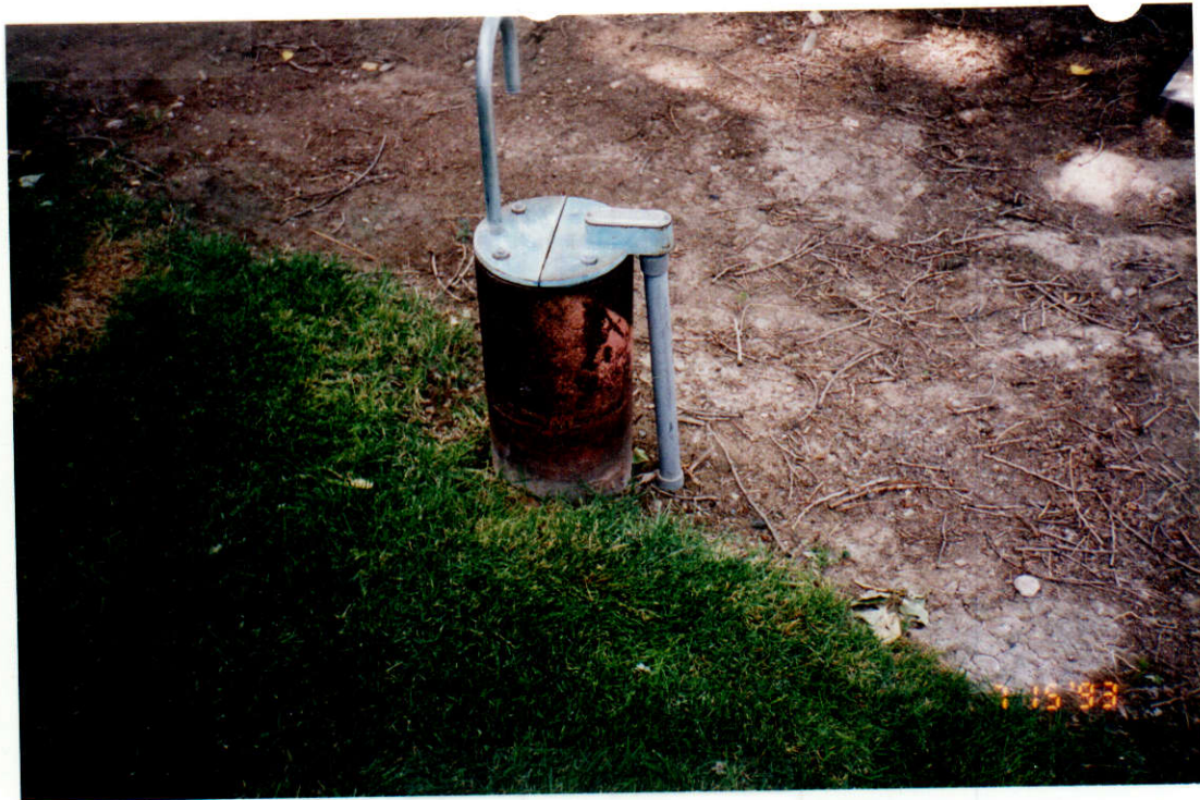
8" well 7.5 HP submersible pump
