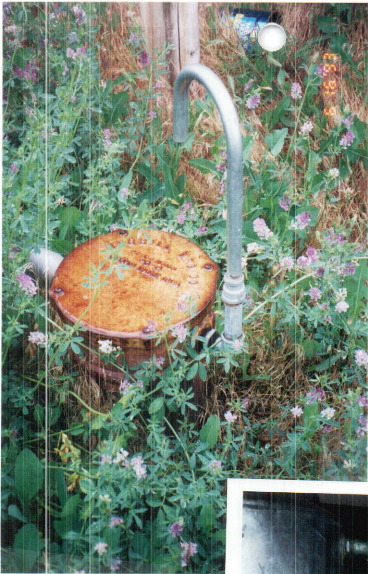
1 8" well 7.5 HP submers pump
