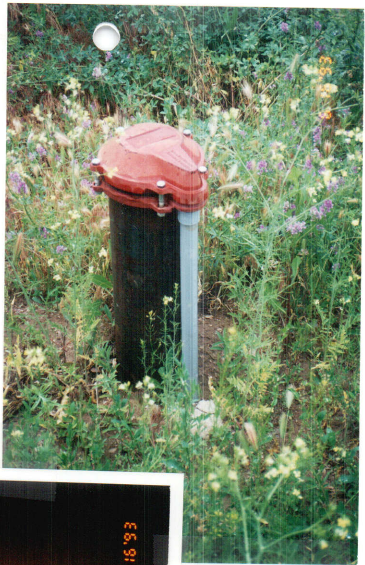
1 6" well 5 HP submers pump
