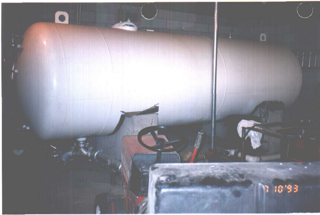
10K gal Pressure Tank
