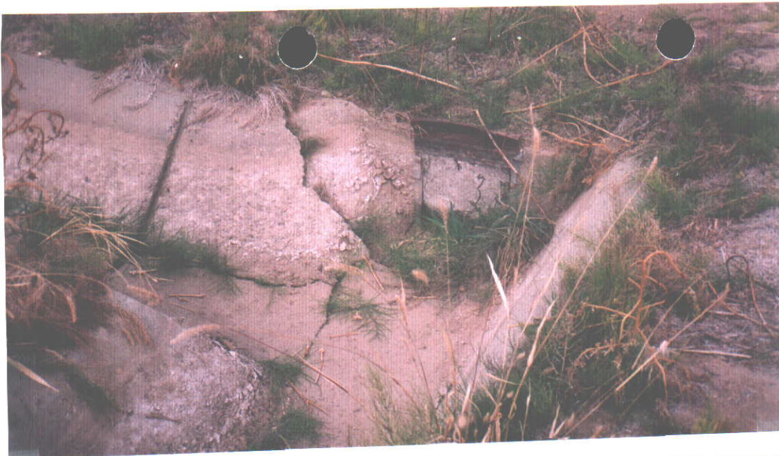
Collection basin and gate to buried pipe
