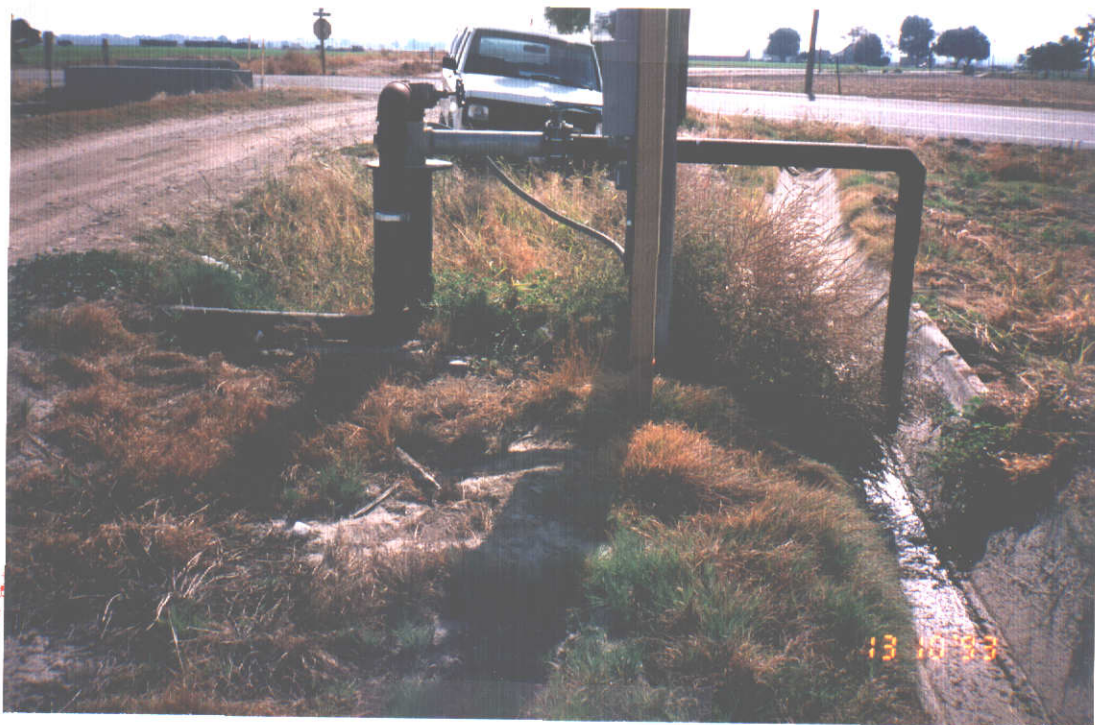
open discharge gravity irrig.
