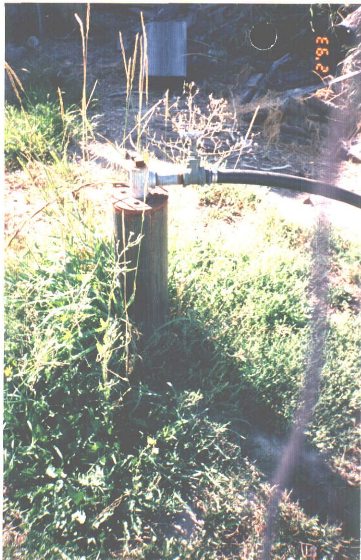
6" well 1 HP submersible pump
