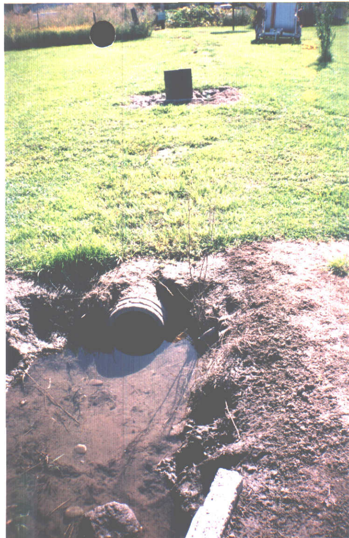
New York Canal water delivery system
