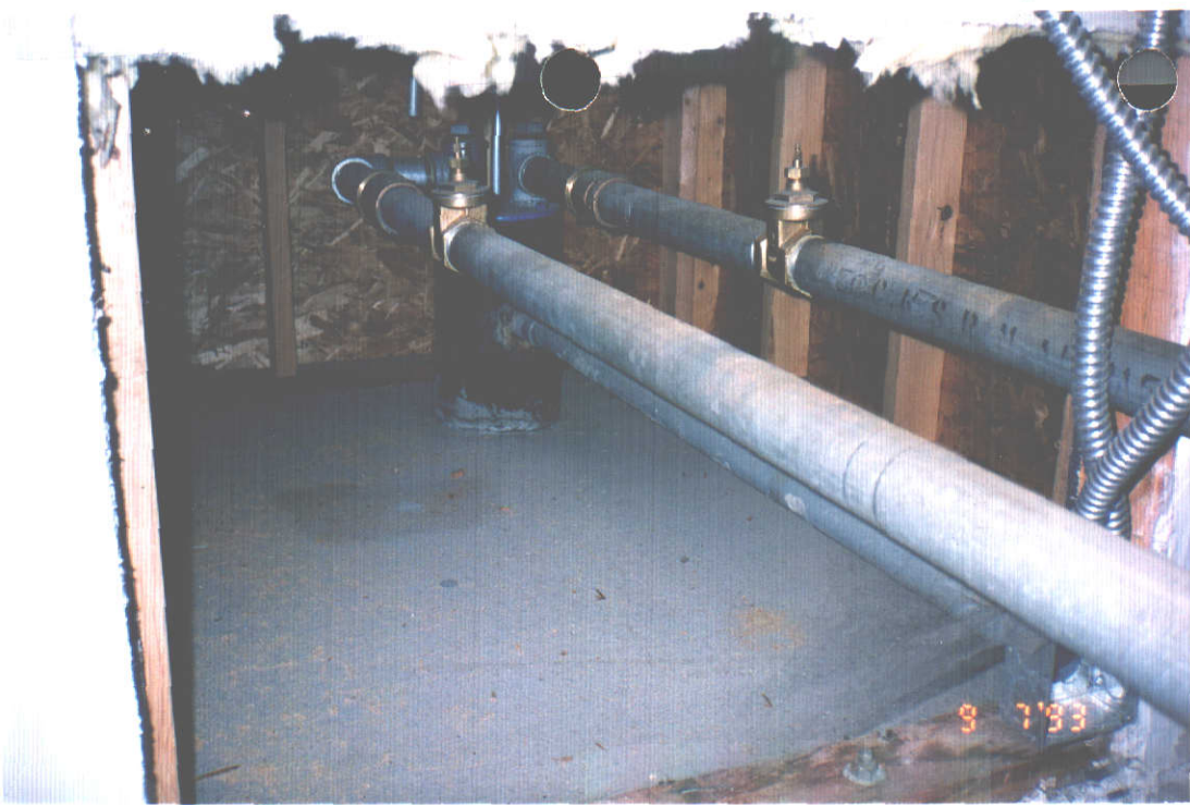
8" well in two 5 HP submersible pumps
