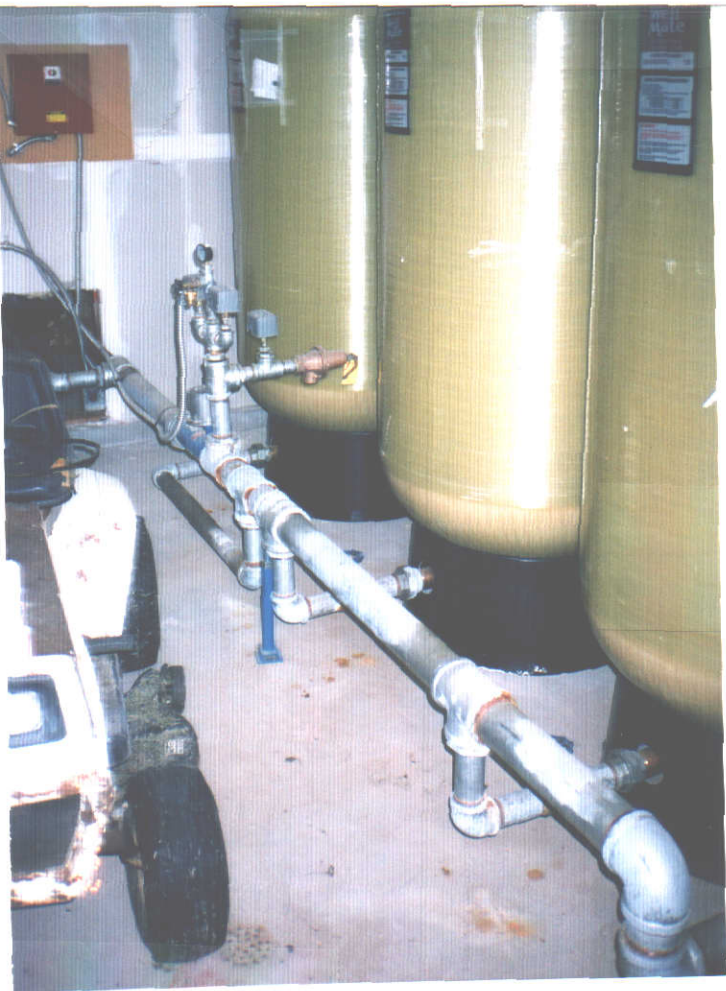
storage tanks + diversion - system
