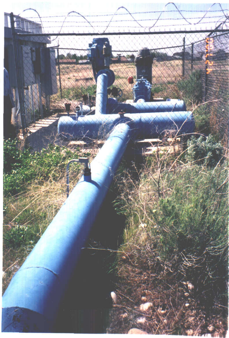
well, pump, booster pump + 1" main- line in SESENE S31 T3N R3E
