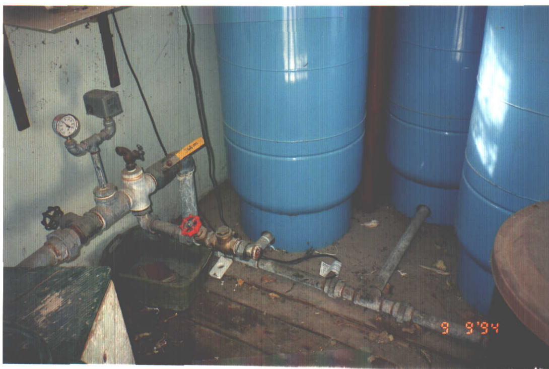
pressure system for powerhouse, restrooms etc.
