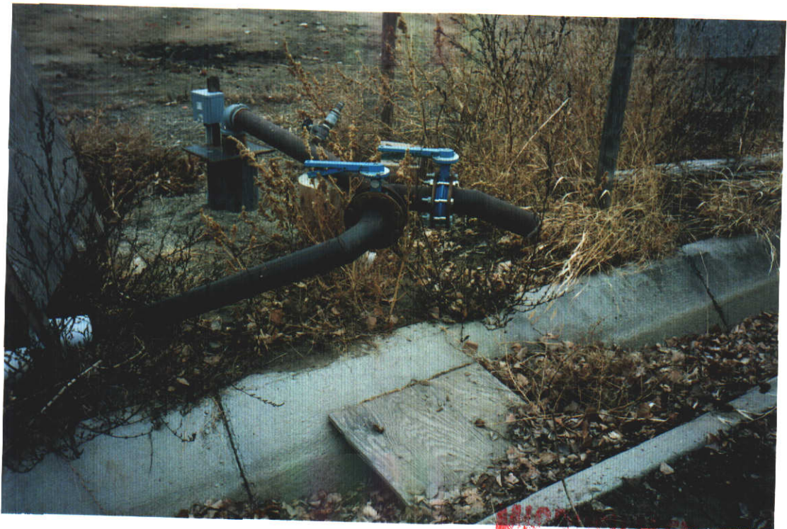
Well and 4" discharge lines. APR 15 1994
