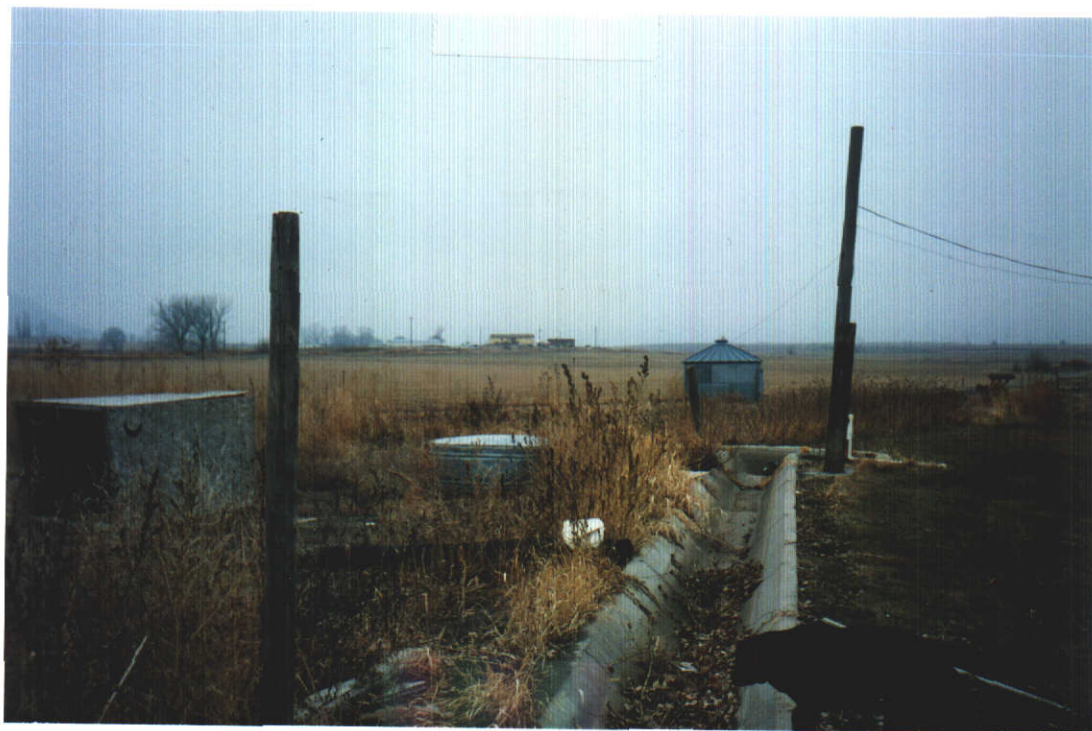
PHOTO THREE- View westerly of bend in concrete ditch and a portion of fields irrigated by system.
