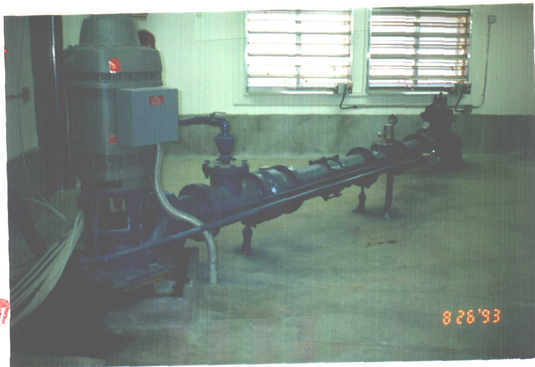
10" discharge system into 12" buried mainline
