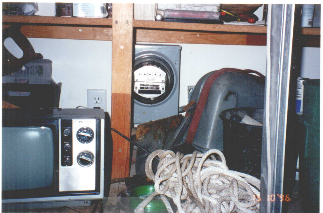
measuring device for well located inside Glen Hickey's garage
