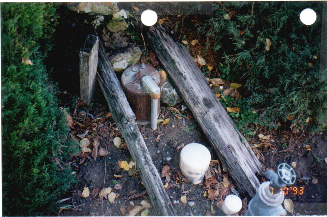
6" well 3 HP submersible pump
