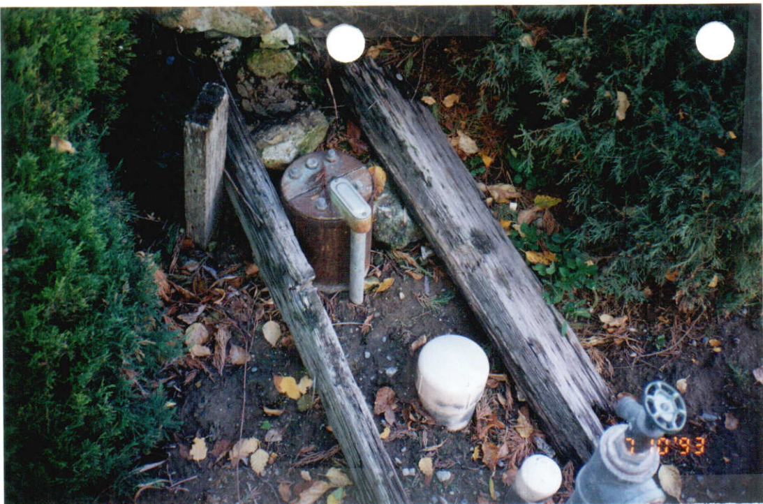
6" well 3 HP submersible pump
