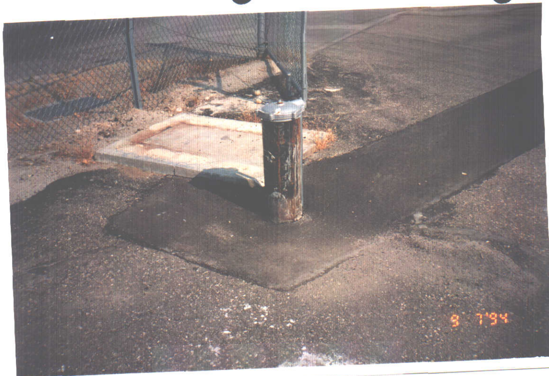
8" well 3HP submersible pump
