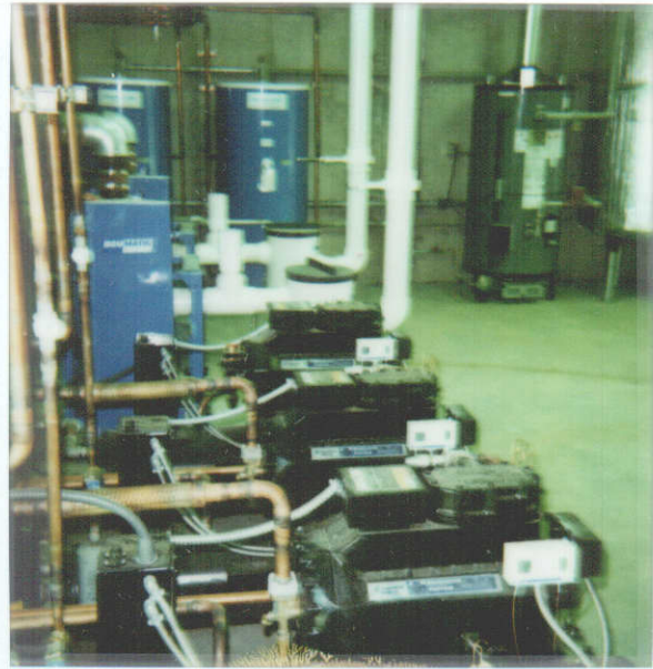
COMPRESSOR & HOT WATER SYSTEM
