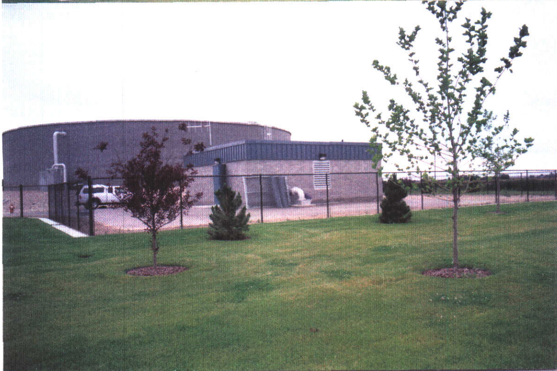
Figure 4. July 16, 2001 photographs of the City of Meridian's #20 municipal supply well pump house. Upper photo looks north from Ustick Road. Green emergency power generator on left behind pump house. Middle view looks east with 2 million gallon Ustick Reservoir in foreground. Lower shot is to the west.
