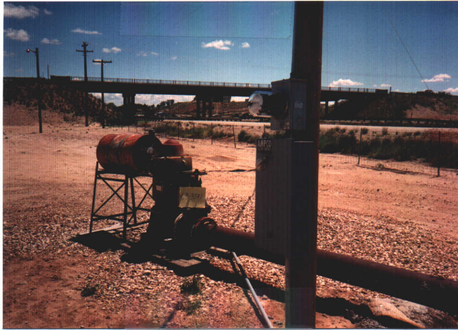
Picture #1 Well head & Pump
