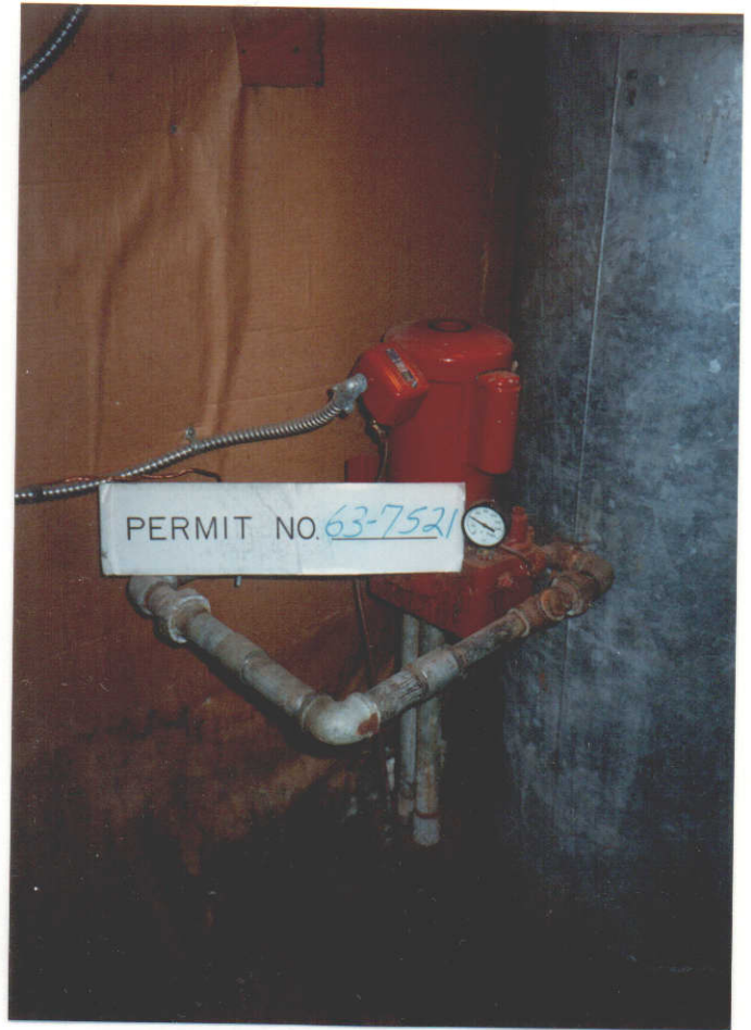
P/D #2 6" casing, artesian well.
