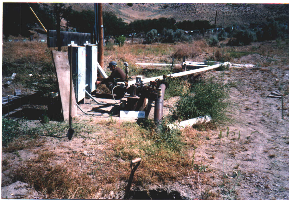
(A) POINT OF DIVERSION TWO SUBMERSIBLE PUMPS ARE SET IN A SINGLE CASING
