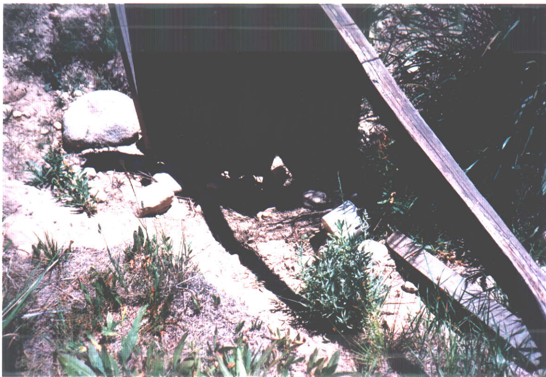
DIVERSION VALVE AT BASE OF DAM. CONTROL LEVER MAY DIVERT WATER TO HAY/PASTURE FIELD BELOW OR TO POND IN FRONT OF LODGE.
