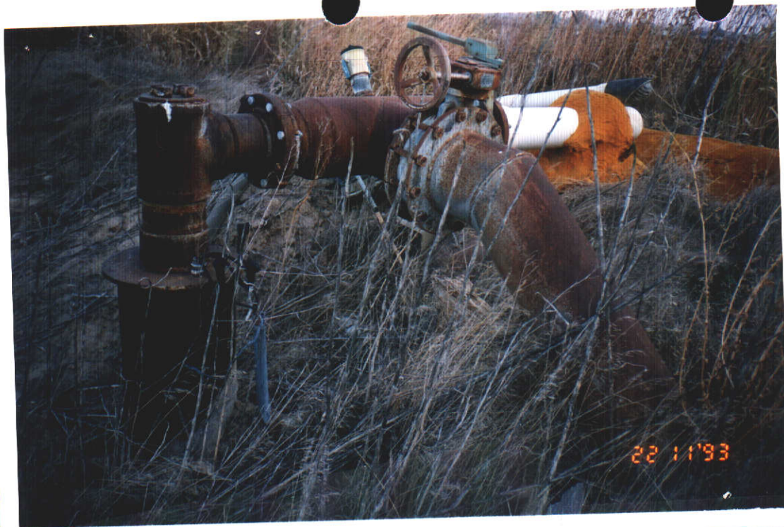
12" well 15 HP submersible pump
