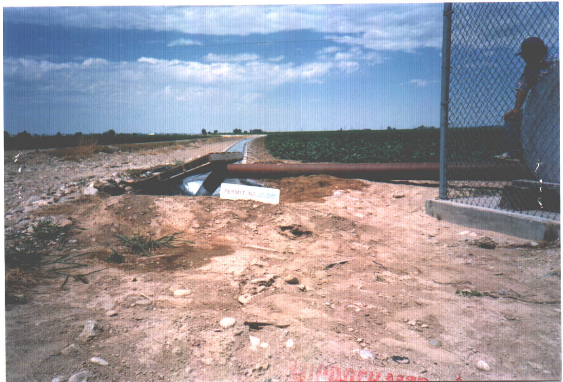
Point of Diversion at right side of photo, ditch system diverts water to place of use in background (looking northwest)
