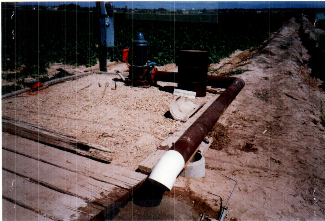
P.D. Looking East. Flow measurement port visible to the right of center.
