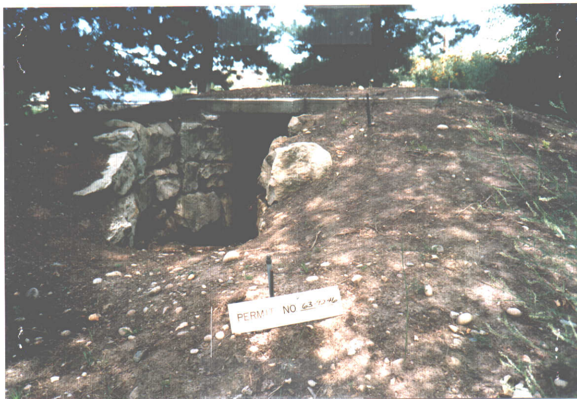
Pumphouse for Well #2 Looking west
