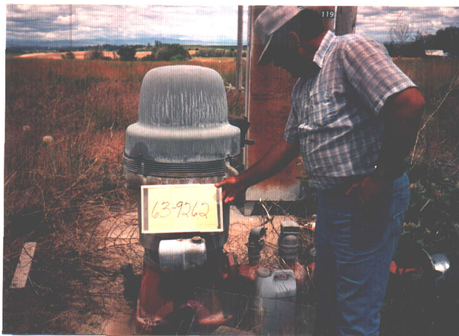
#1 Pump motor and well site
