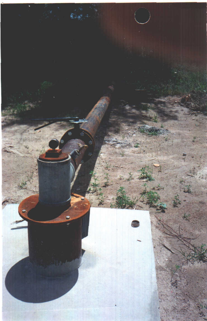
12" well 25 HP submersible pump
