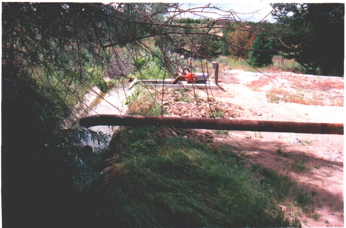
open discharge (Booster pump in background)
