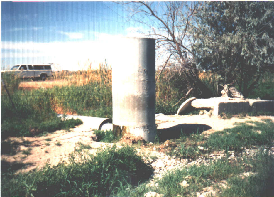
#2 Collection tower that receives water from a buried 12" pipe prior to delivery under Hwy 20-26 to the P/U. This tower is located North of the highway.
