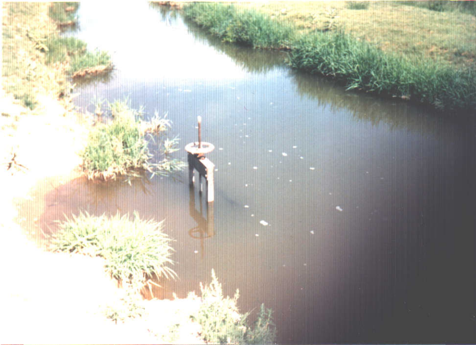
#1 P/D and headgate in the Canyon Canal
