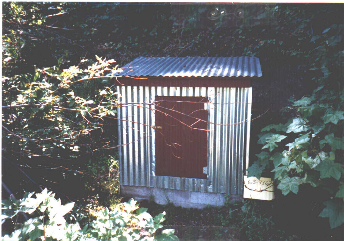
P.D. Collection box with protective structure at Spring Looking WSW
