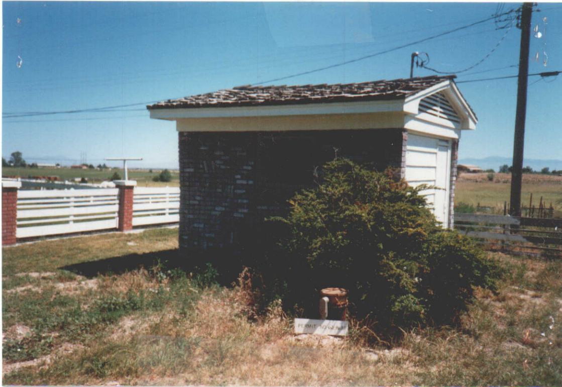
P.D. Well #2 Brick and wood pumphouse 10' x 12' Looking Northeast Well #2 is visible in lower right center
