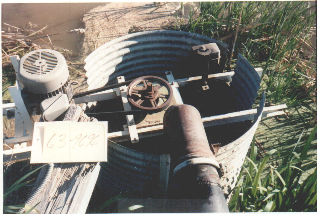
#1 Point of Diversion and pumping system.
