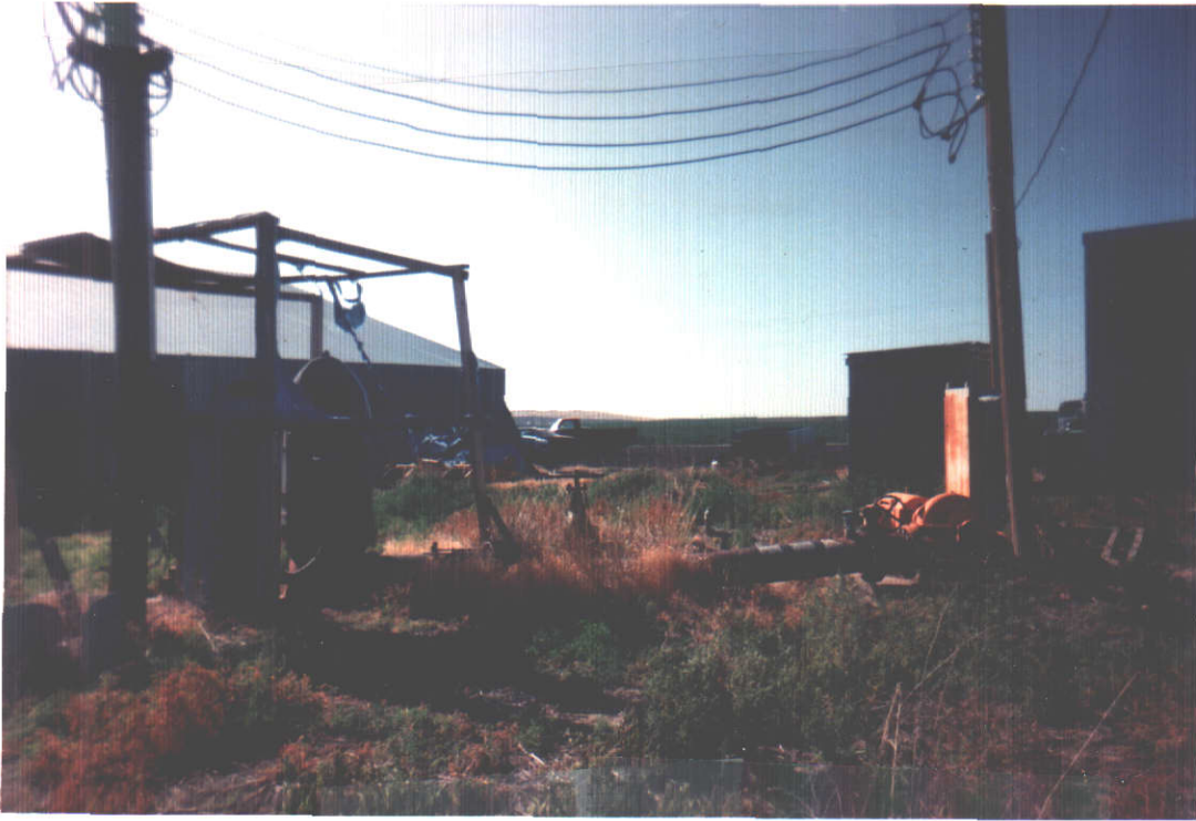
View of well & booster unit.
