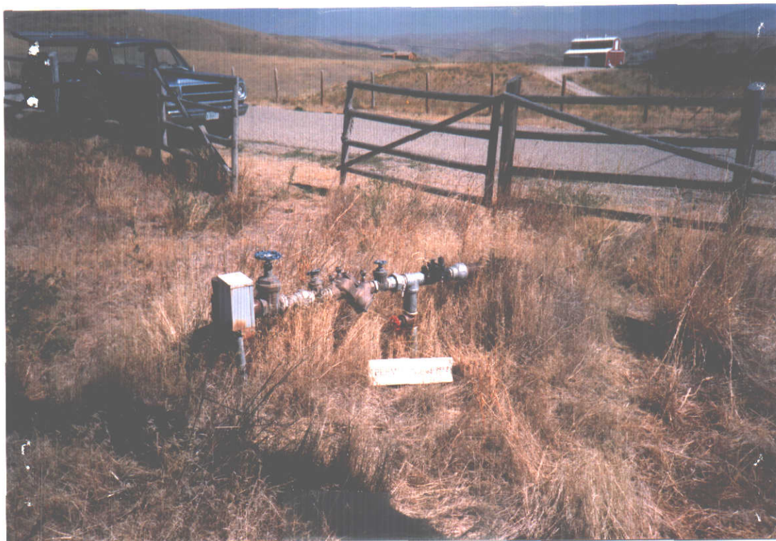
P.D. looking North east The well is behind the electrical box
