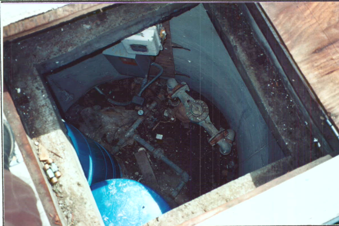
7 1/2 hp well House
